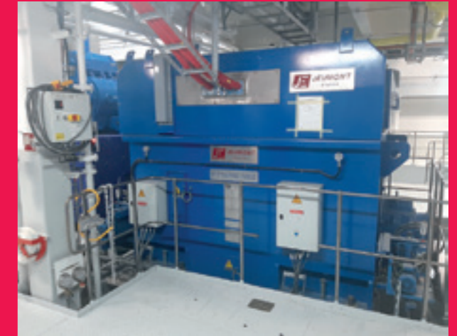
Ferry propulsion system
