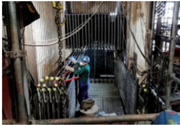
Lyon metropolitan authority waste-to-energy plant, Rillieux-la-Pape, France
