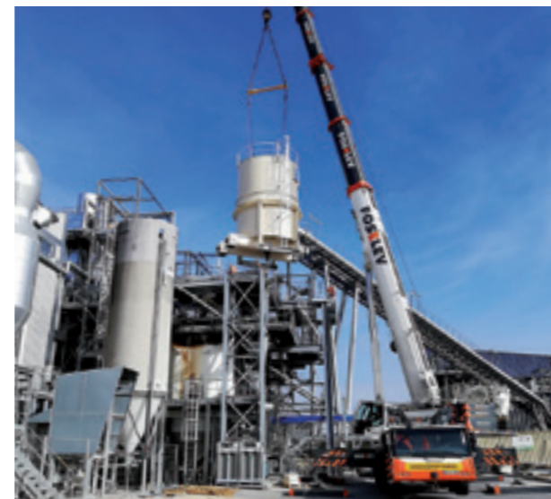
Cristal Union gasifier, Bazancourt, France
